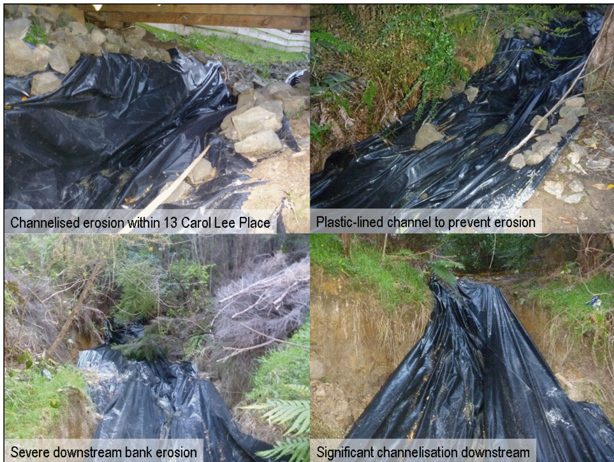
Figure 10: Photos taken during site visit on 9 Sep. 2011, illustrating severe downstream erosion
