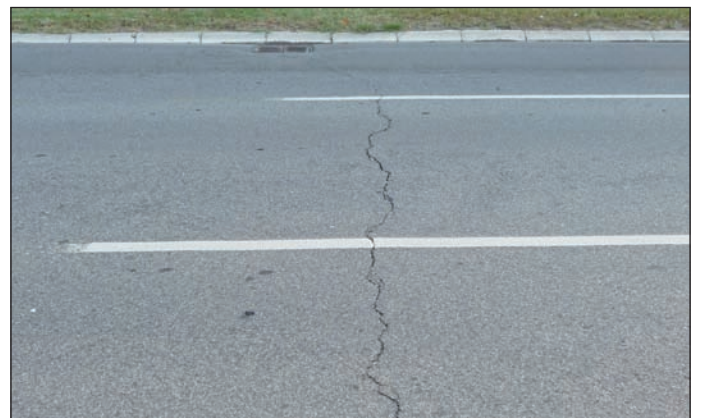
Reflective crack in an asphalt surface course
