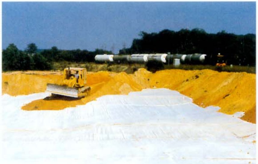
Once installed, the fabric was strong enough to give support to 4 t bulldozer laying fingers of fill material during the initial fill process.
